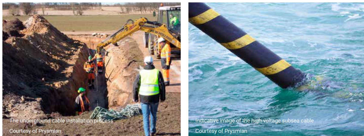
Figure 5 – The underground cable installation process and an example image of an HV subsea cable
